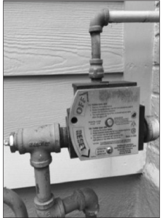
A NATURAL GAS SAFETY VALVE
