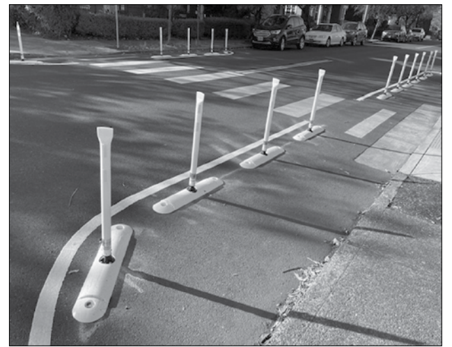
BUMP OUTS WERE INSTALLED ON NE FREMONT IN MID-NOVEMBER. PHOTO COURTESY OF JOHN SANDIE, BWNA.
