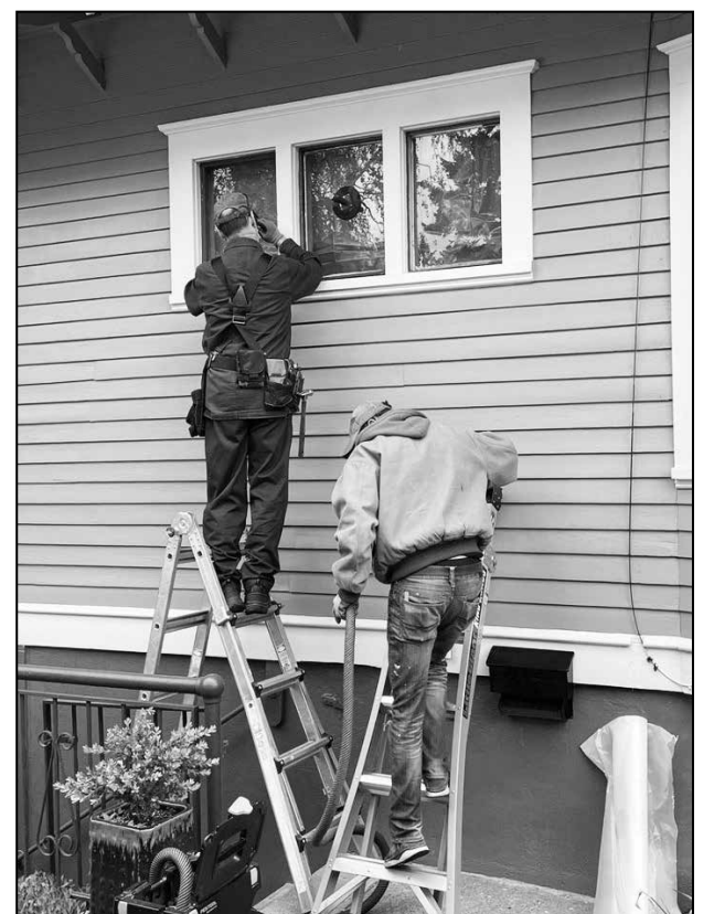
THE SASHWRIGHT CO. TEAM PREPARES TO REMOVE THE CLEAR GLASS PANES THAT WERE PUT IN PLACE WHEN THE ORIGINAL WINDOWS WERE REMOVED IN THE 1970S.
