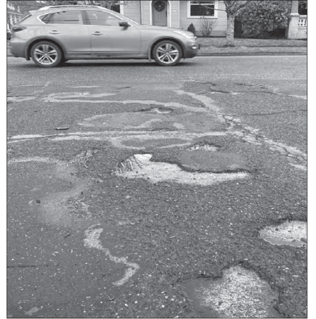
RESIDENTS CAN CALL THE PBOT POTHOLE HOTLINE AT 503-823-BUMP TO REPORT POTHOLES. THE CITY APPRECIATES HEARING ABOUT DEVELOPING PROBLEMS BEFORE THEY REQUIRE MORE COSTLY REPAIRS.
