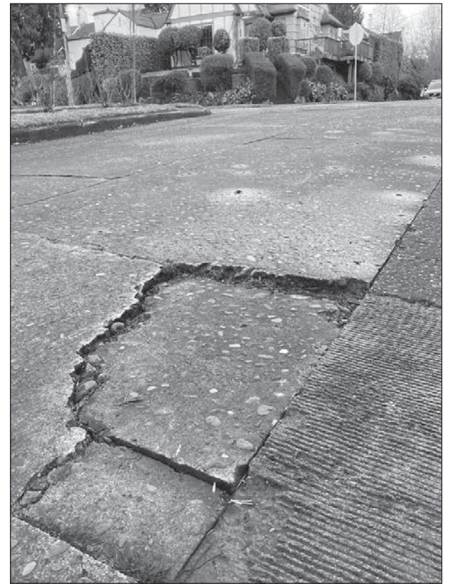
UNEVEN SURFACES COMPOSED OF VARIOUS PAVING MATERIALS CREATE POTHOLE HAZARDS IN ALAMEDA.
