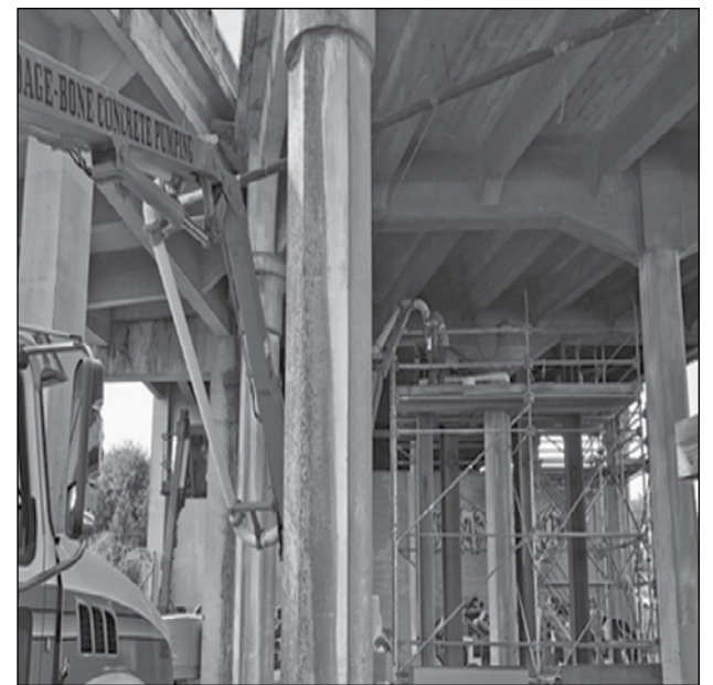
CEMENT IS POURED AS WORK IS COMPLETED ON NE 33RD AVE. BRIDGE.
